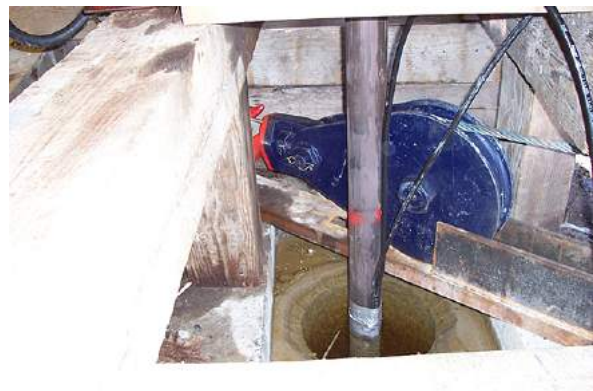
Sheave wheel for 3/4 inch safety cable at collar of drill hole with packer inflation hoses attached to HQ drill rods
