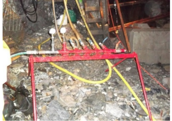
Four-way header for cement grouting
