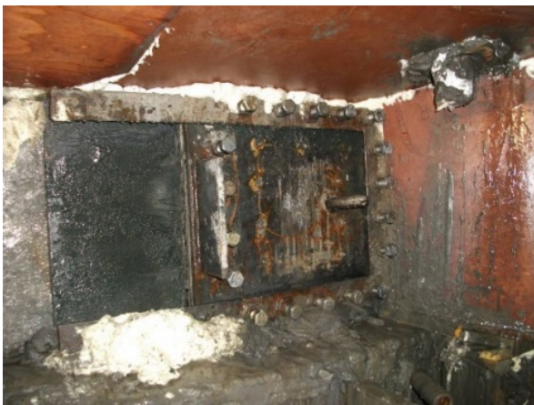
Water control gate in closed position
