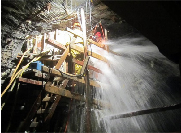
Workers closing a water control gate to stop a 1,500 GPM water inflow
