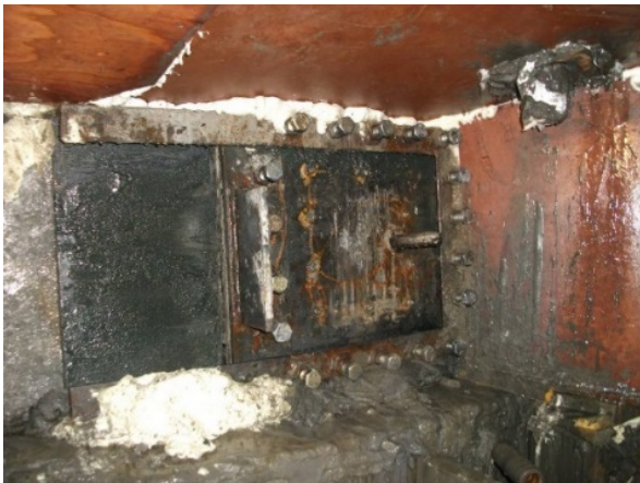
Water control gate in closed position
