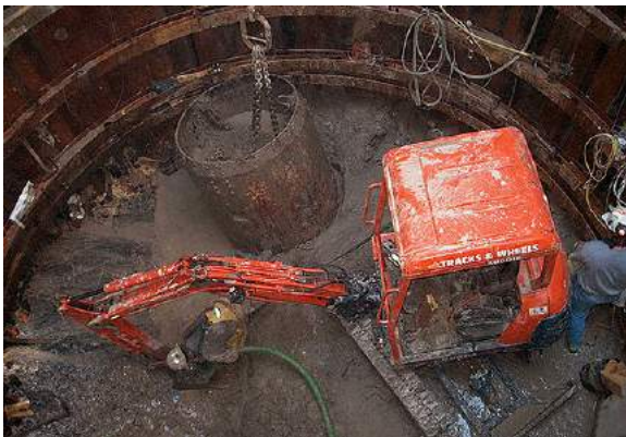
Quicksand inflow at the bottom of the shaft
