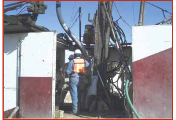
Excellon Resources, Platosa Mine, Mexico Deep hole drilling and high-volume cement grouting operations were used to seal water-bearing rock formations and successfully recover a flooded underground silver mine.
